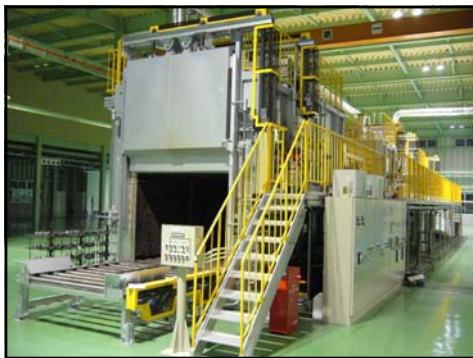
Solution Furnace with open front door.
