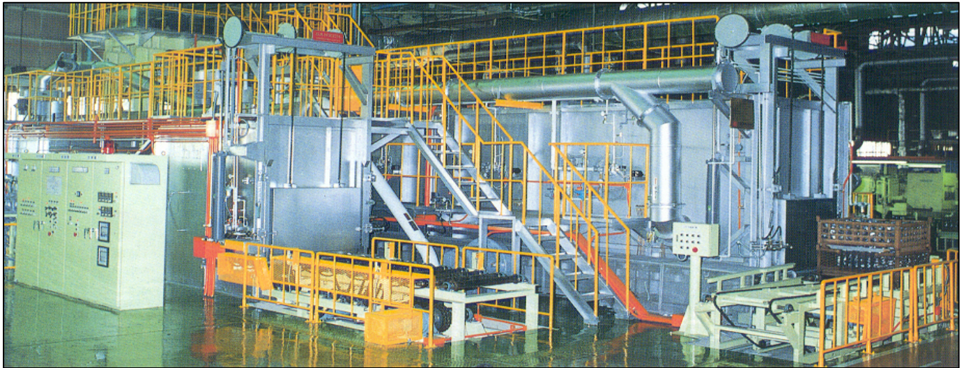
T6 Heat Treatment Installation provided with loading and unloading tables.
