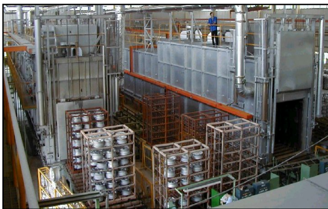
General view of T6 Heat Treatment Installation based on "U" type arrangement.
